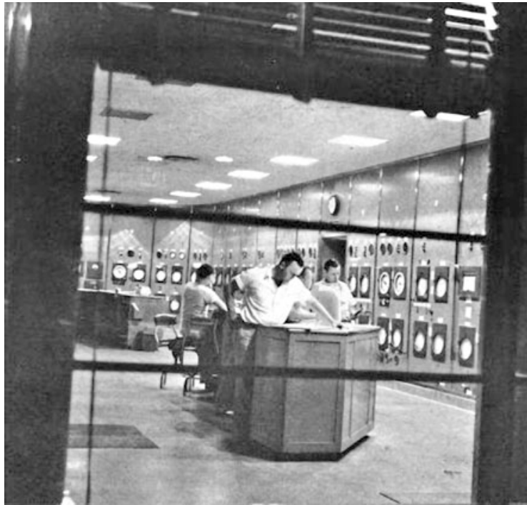
Fig. 3 Cat Cracker Control Room, Shell Oil Deer Park Refinery. Credit United Steelworkers Local 13-1, Pasadena, Texas.
